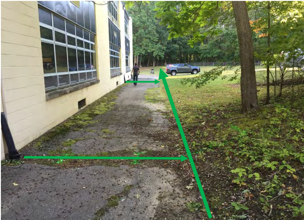
The photo above shows an area where multiple roof drains tie into the main trunk, the flow of the roof drains can be seen by the green arrow.
