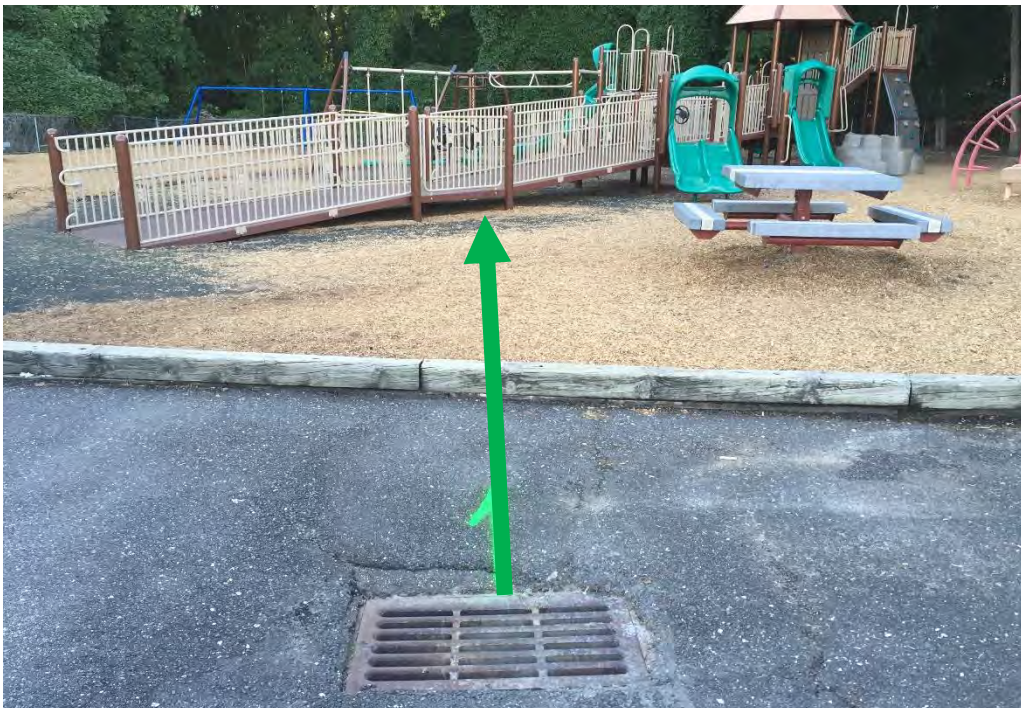
The photo above shows the path the storm drain follows. This drain runs through the playground and dumps out beyond the fencing.
