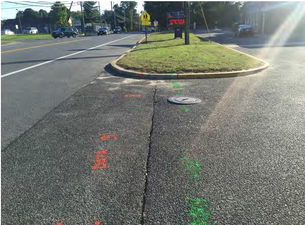
The photo above shows a data line and a sewer line. The data line was approximately 3' subsurface while the sewer line was located at approximately 12' +/-.
