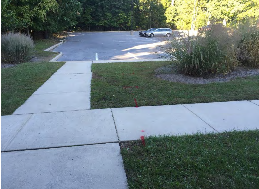
The photo above shows the path the conduit takes for the site lighting located in the photo.
