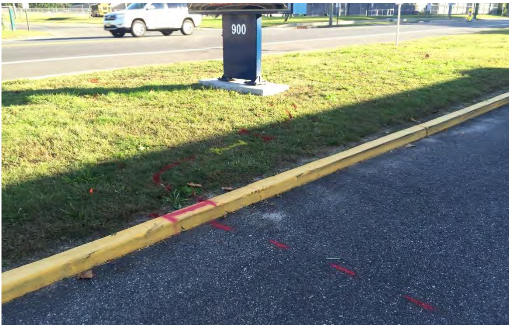
The photo above shows the same gas and electric lines as mentioned in the previous photo. The electrical lines were located going to the sign for the school. The gas line was located up to a valve on the shoulder of Gibbsboro road.
