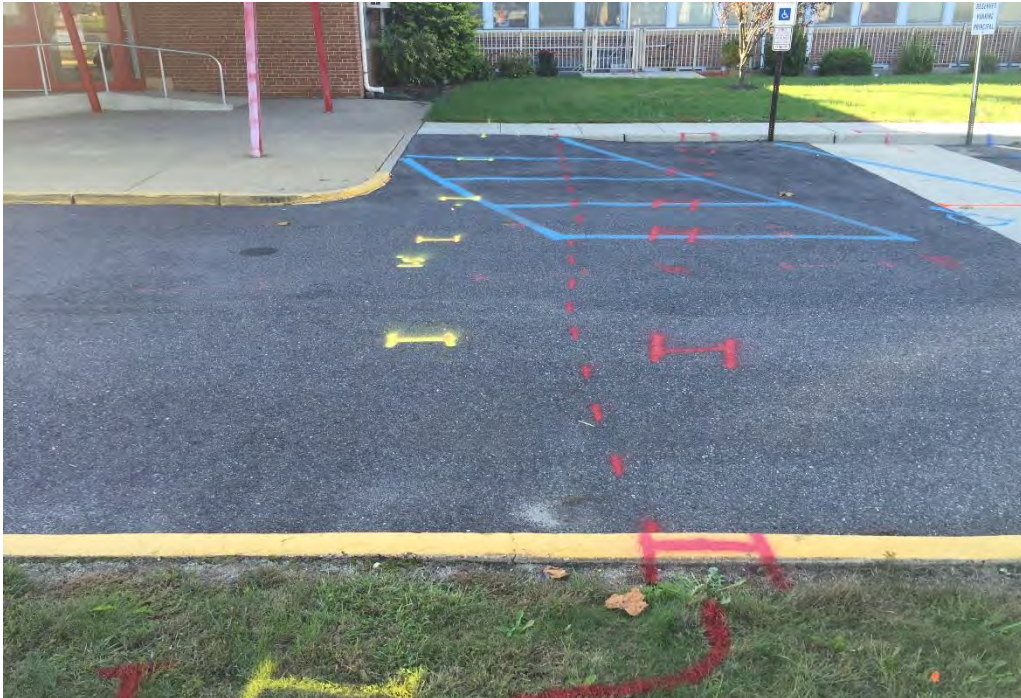
The photo above shows multiple electric lines that were located utilizing the RD7000. These lines are marked in red marking paint. The gas line can be seen marked in yellow located at approximately 2'.
