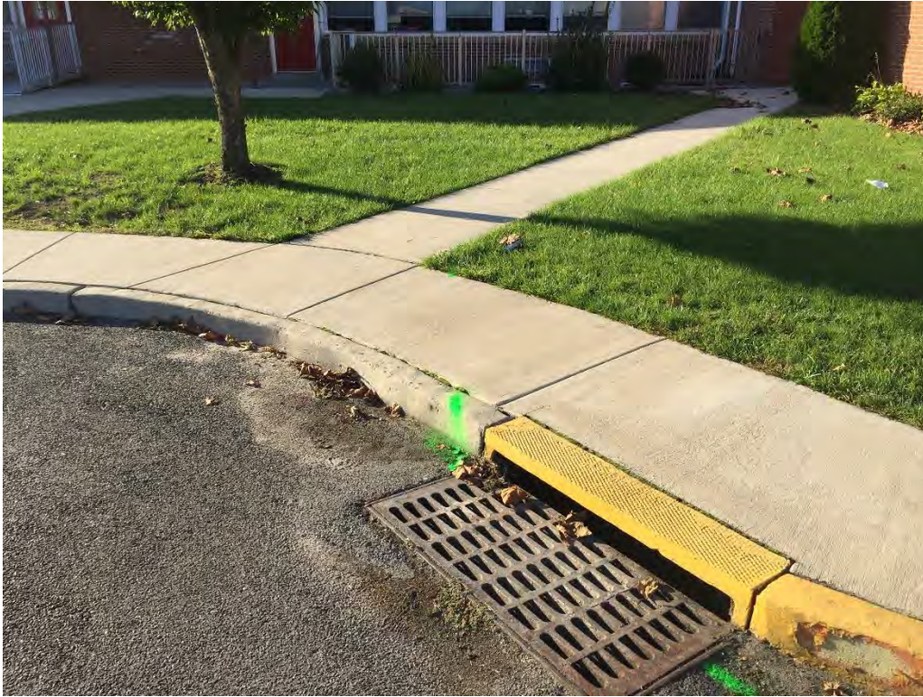
The photo above shows where the roof drains that ran parallel to the building tie into the storm drain.
