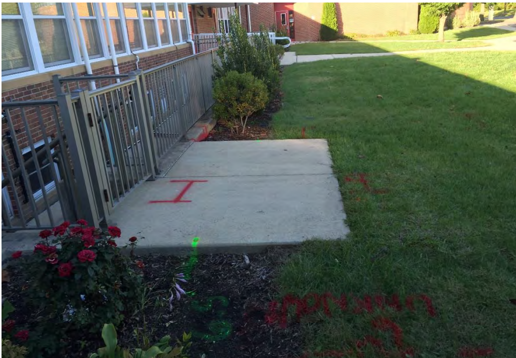
The photo above shows multiple locations where the live electric enters the building. The path of the roof drain/storm runs parallel to the fence.
